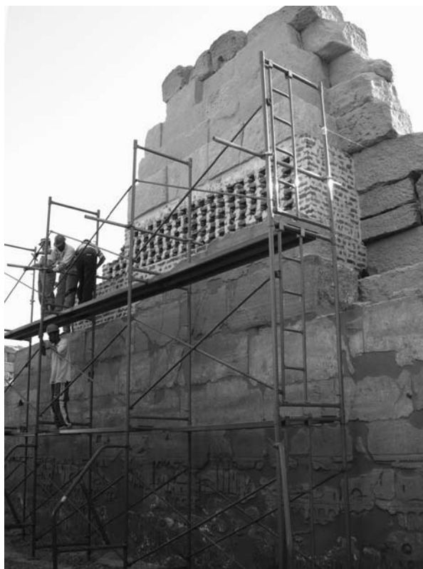
Brick buttress built against projecting eastern wall section of the Colonnade Hall, Luxor Temple, view from the south, showing four levels of veneer blocks and below, the brick matrix into which the Khonsu Barge fragment group will be inserted. Dany, Mustafa, Saber, and Sayid. Photo by Ray Johnson
