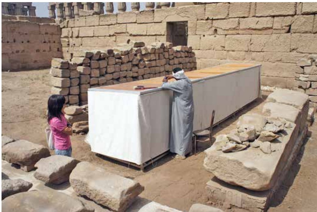
Figure 13. Hiroko supervising installation of “hospital” mastaba new cloth and roof copy (photo by Ray Johnson)
