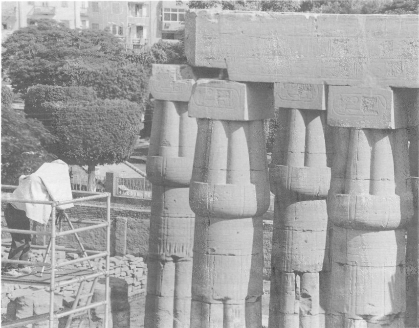
Figure 6. Balanced on the aluminum scaffold, photographer Cecile Keefe takes documentary shots of the architraves of the sun court of Amenhotep III at Luxor Temple
