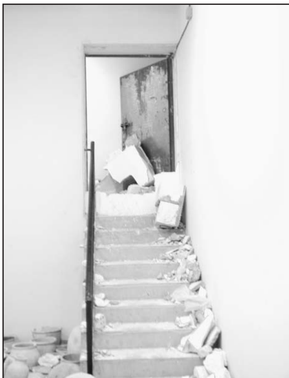
Iron door to basement storage and protective block wall penetrated by looters between April 10 and 11. Iraq National Museum
