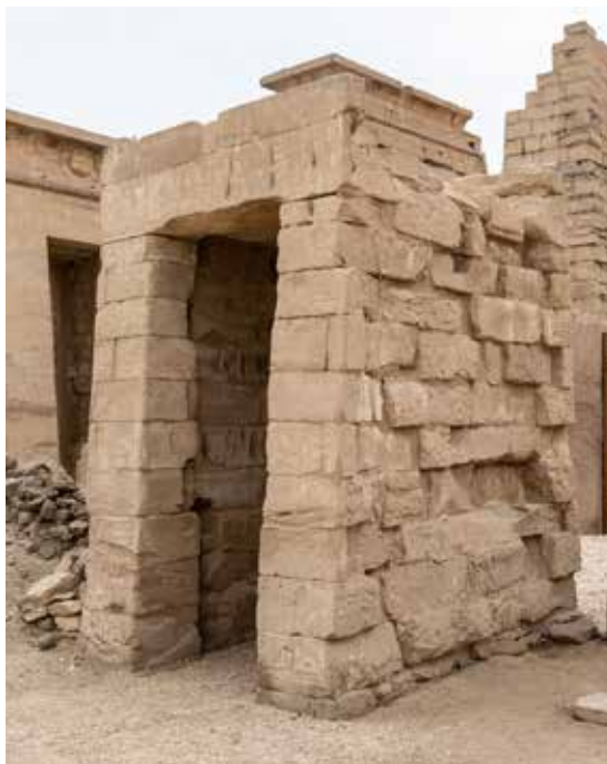
TOP: Figure 17. Taharqa gate March 2020 before intervention. Photograph by Frank Helmholz.
