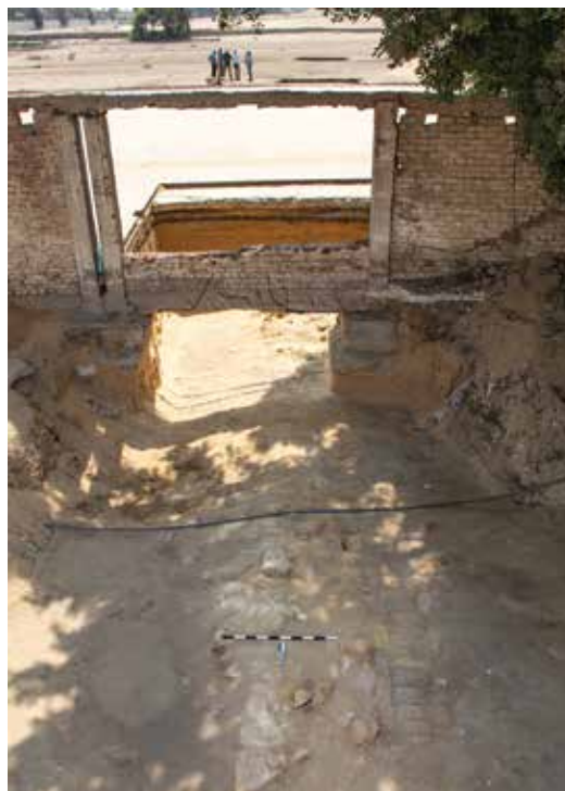
Figure 3. The west RAB wall continuing below the Abu Hol Sports Club; view to the south.
