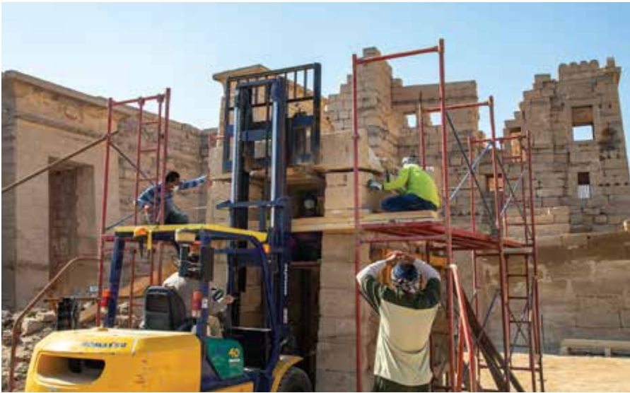
Figure 10. Removing the lintel block of the Taharqa Gate, January 2022. Photo by Frank Helmholz.
