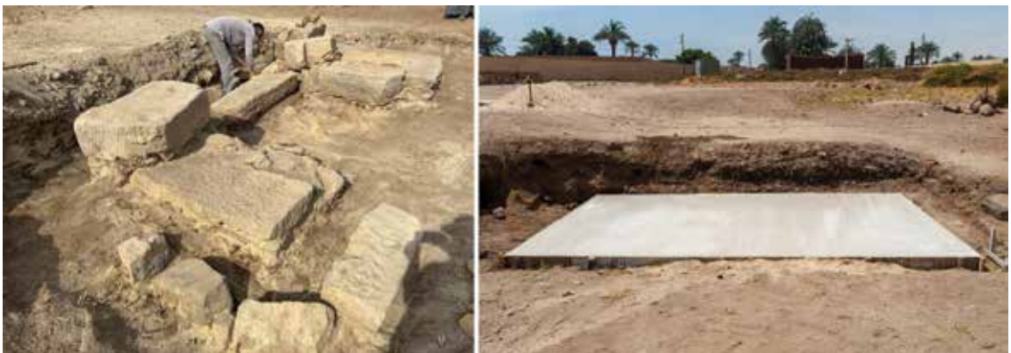
Figure 9. Left , Claudius Gate foundation before dismantling, January 2022. Right , new subfoundation slab, April 2022. Photos by Frank Helmholz.
