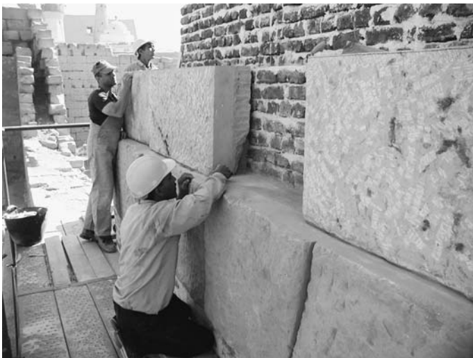
Figure 11. Laying sandstone veneer over brick buttress, Colonnade Hall, Luxor Temple, looking toward the north; Dany Roy, Ali Mahmoud, and Saber Ahmed Taya. Photo by Ray Johnson
