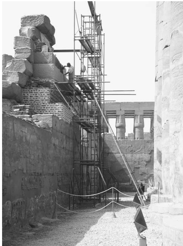
Figure 9. Brick buttress built against projecting eastern wall section of the Colonnade Hall, Luxor Temple, view from the north; Dany Roy. Photo by Ray Johnson
