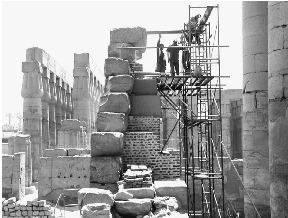
Figure 12. Brick buttress with sandstone veneer built against projecting eastern wall section of the Colonnade Hall, Luxor Temple, view from the north. Hassan Yousef Aly, Dany Roy, Saber Ahmed Taya, and Ali Mahmoud. Photo by Ray Johnson
