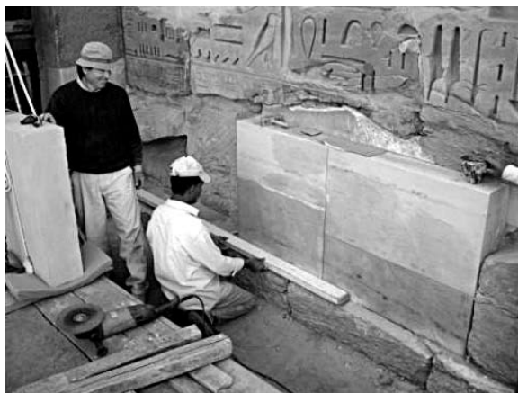
Frank and Saber inserting patch stones into the northern outer wall of the Small Amun Temple sanctuary. Photo by Ray Johnson
