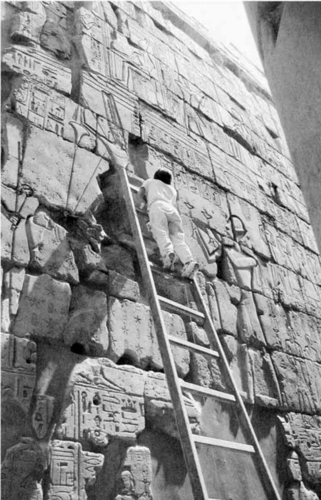
Conservator Hiroko Kariya installing a plumb bob monitor on the south face of the east pylon, Luxor Temple
