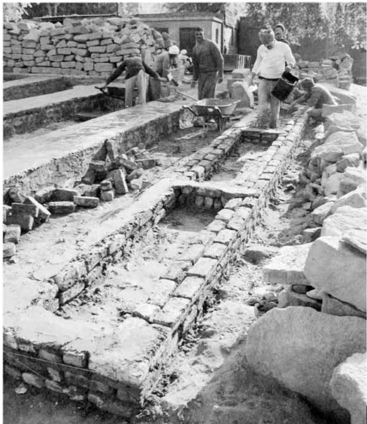
Workmen constructing damp-coursed brick mastaba platforms for decorated wall-fragment storage and analysis, Luxor Temple blockyard
