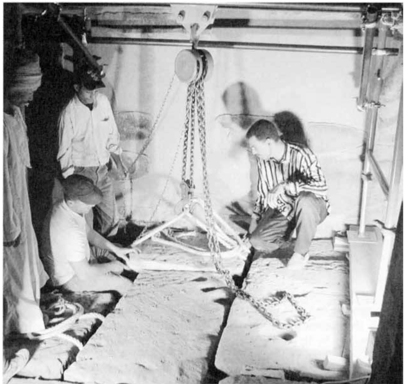
Stonecutter Dany Roy supervising the removal of floor blocks in the naos room of the small Amun temple, Medinet Habu
