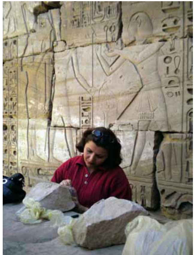
Inspector Ghada drawing a loose block at Khonsu Temple
