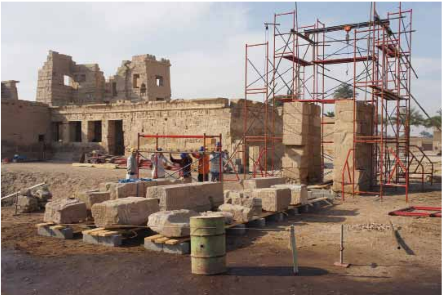
Medinet Habu Domitian gate dismantling March, 2011. Small Amun temple and Ramesses III High Gate on the left
