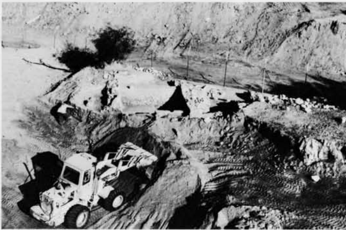
Donald Whitcomb and a front-end loader remove clean sand from around the 1988 J area excavations.
