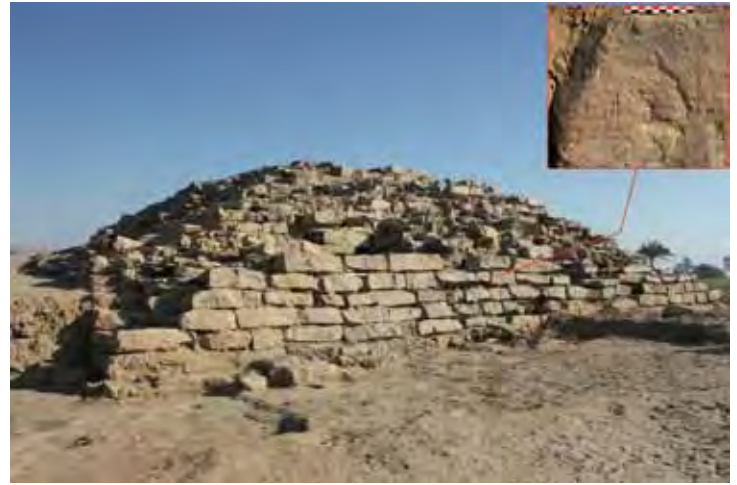
Figure 10. South face elevation and graffiti position
